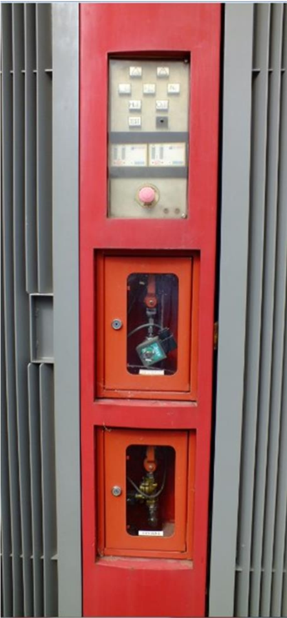
Figure 70 : Emergency shutdown and h2/o2 valves on an AREVA green box ©AREVA/ENSOSP 2015
