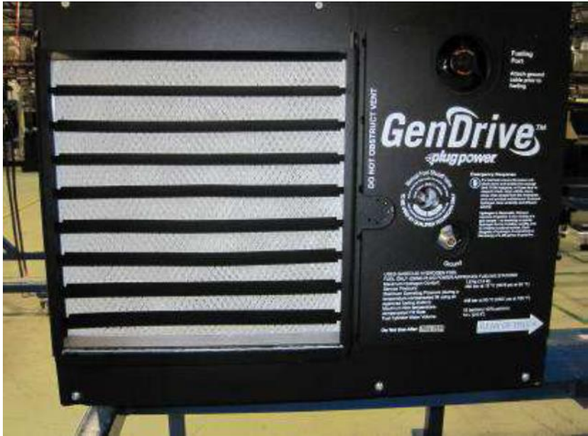
Figure 49. Forklift H2 release vent (on each side) ©Air Liquide-2014
