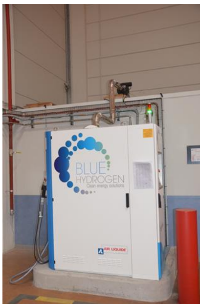
Figure 37 : Indoor refuelling station for forklift (dispenser)
