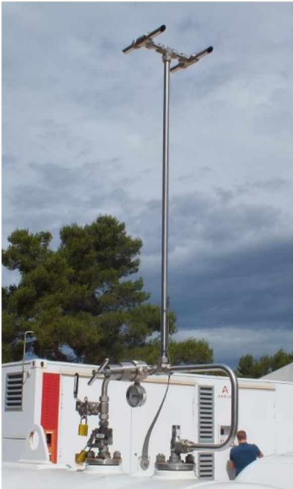
Figure 67 : Areva backup System (pressure release devices) ©AREVA/ENSOSP 2015
