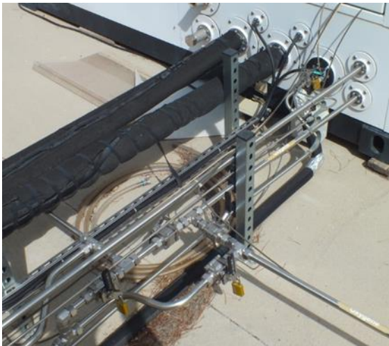
Figure 69 : Areva backup System (H2 and O2 network detail with valves) ©AREVA/ENSOSP 2015
