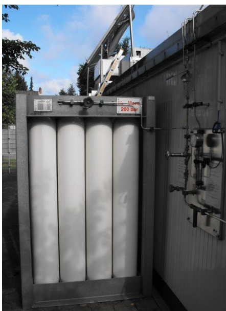
Figure 38 : Refuelling station low pressure storage 200 bar
