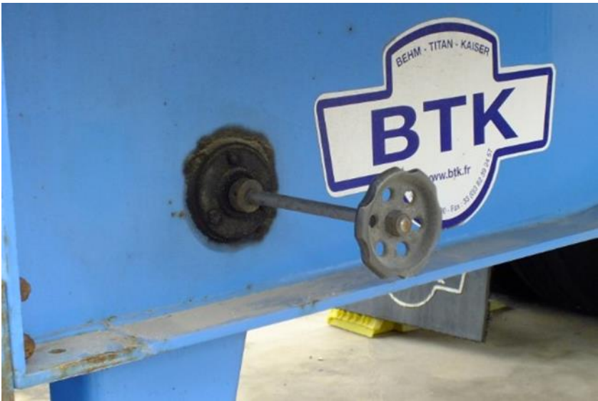
Figure 56 Trailer Main H2 valve (outside view) © Areva/ENSOSP 2015
