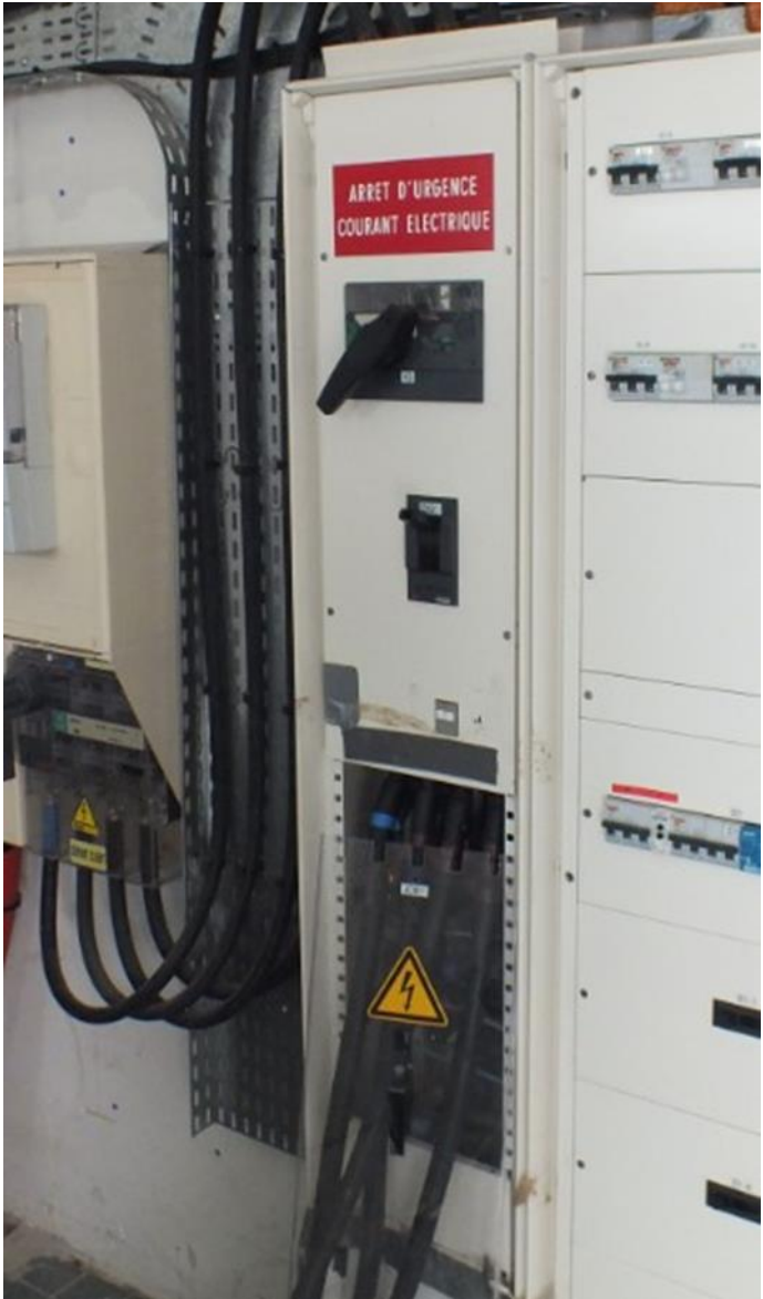
Figure 59 : Main electrical Emergency Shutdown © Areva/ENSOSP 2015
