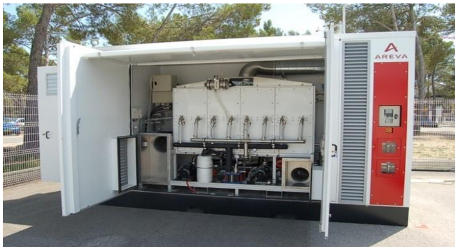
Figure 14: Fuel cell backup power coupled to the IP Energy data center.
