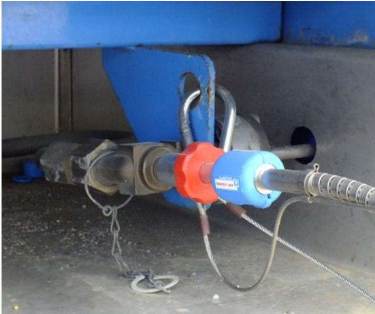
Figure 57 : Trailer Main H2 valve (inside view) © Areva/ENSOSP 2015
