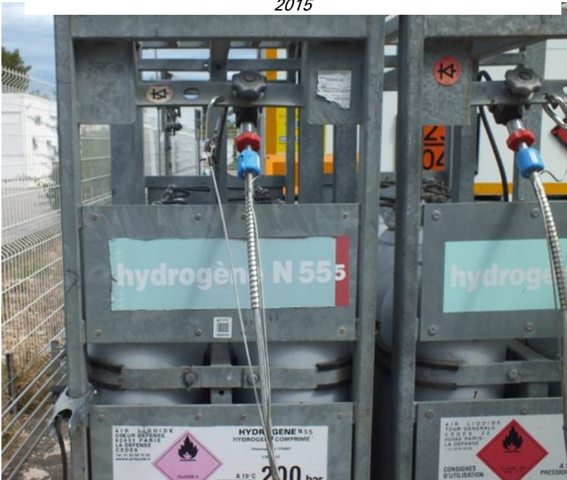
Figure 58 : Valves on a H2 bottles Rack © Areva/ENSOSP 2015
