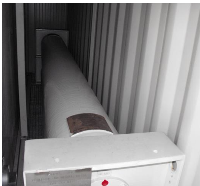
Figure 39 : refueling station high pressure storage 1000 bar
