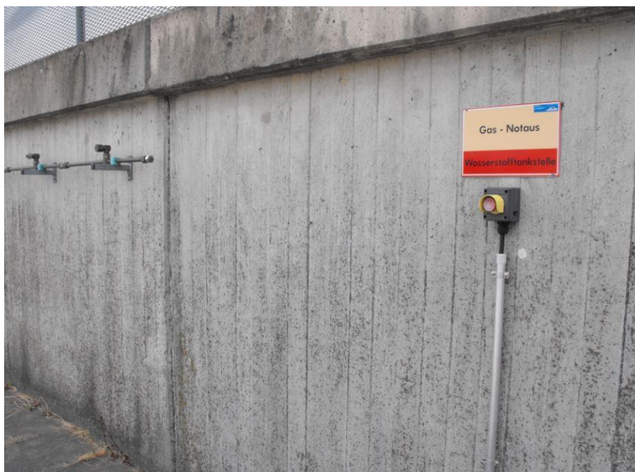
Figure 40 : Refueling station ESD away from dispenser (Hamburg airport)
