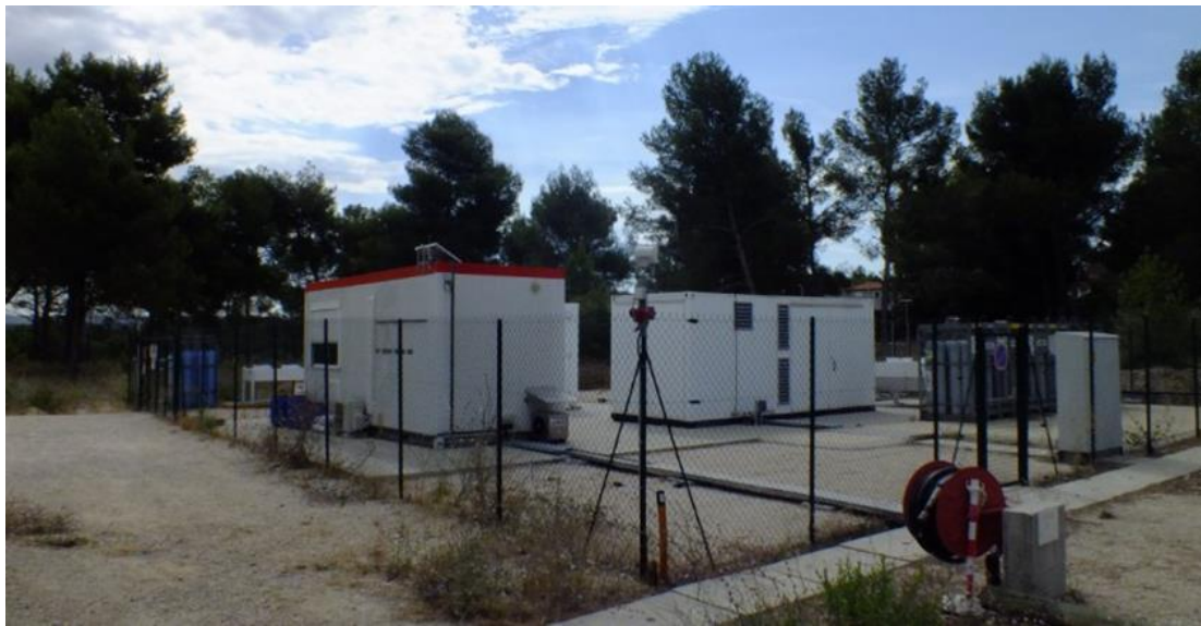
Figure 64 : Areva backup System global view ©AREVA/ENSOSP 2015
